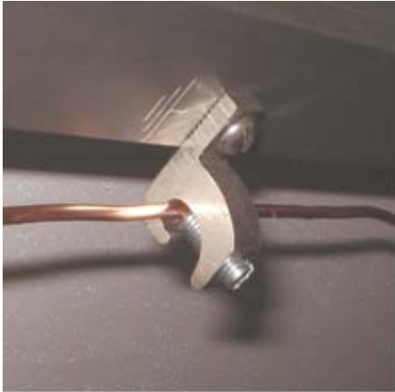
Grounding Lug Picture
